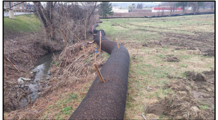
Figure 7: Filter sock used to provide erosion and sediment control (Source: Westmoreland Conservation District)
