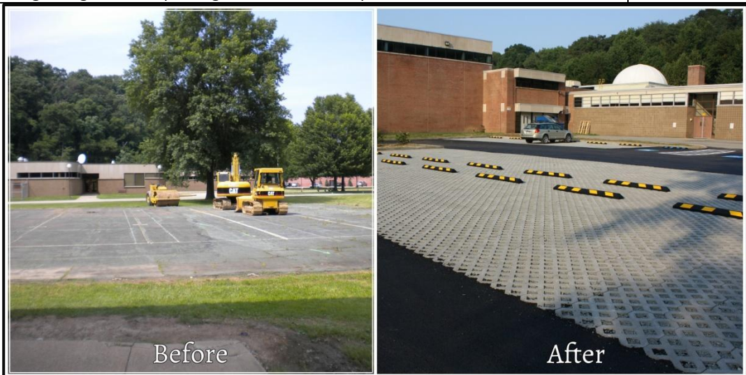
New parking at Valley High School with permeable pavers. Photos: Westmoreland Conservation District
